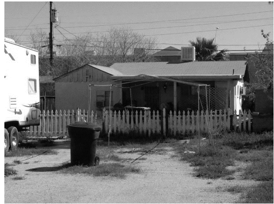
Property is unmaintained and the covered carport has been partly removed, but not entirely and is in need of significant repairs.
